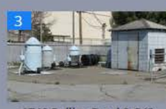
1740 Rollins Road & 842 Cowan Pump Station
