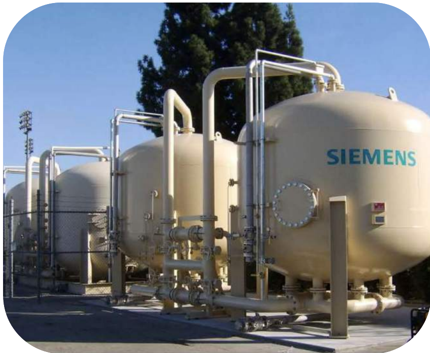
Figure 10: Typical GAC Vessels
