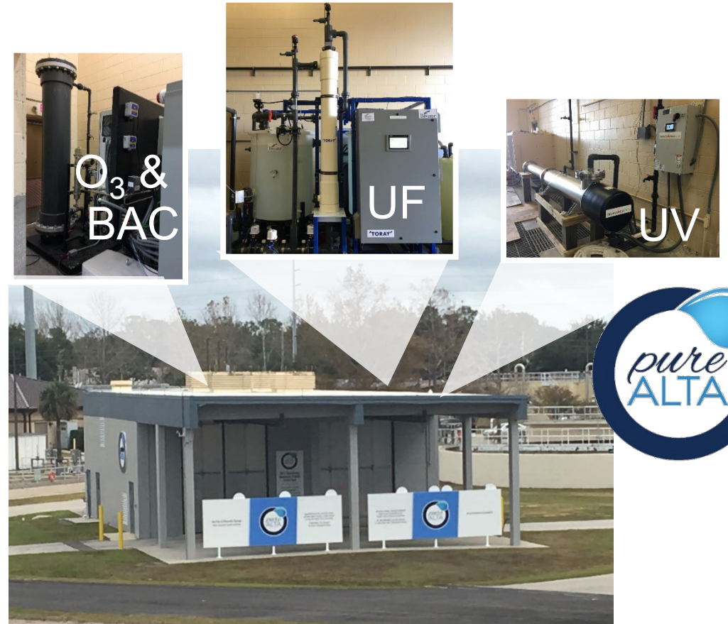
CITY OF ALTAMONTE SPRINGS (FLORIDA) DEMONSTRATION AWPF
