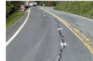
The 9 slides from 2022-23 storms do not include known vulnerabilities at other road sections.
