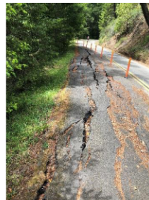
Road damage from 2021 storm, still in need of permanent repair.
