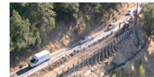
Sides have caused the road to close to one-lane in several locations, limiting emergency access.
