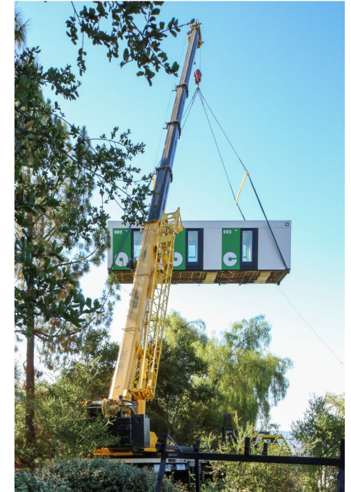
Fire-resistant, steel-framed, High ceilings...and meet codes
